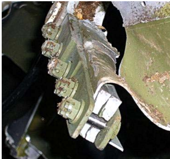
Figure 3 – Location of fracture of the lower spar cap of the left wing with visible outermost close-tolerance bolt
