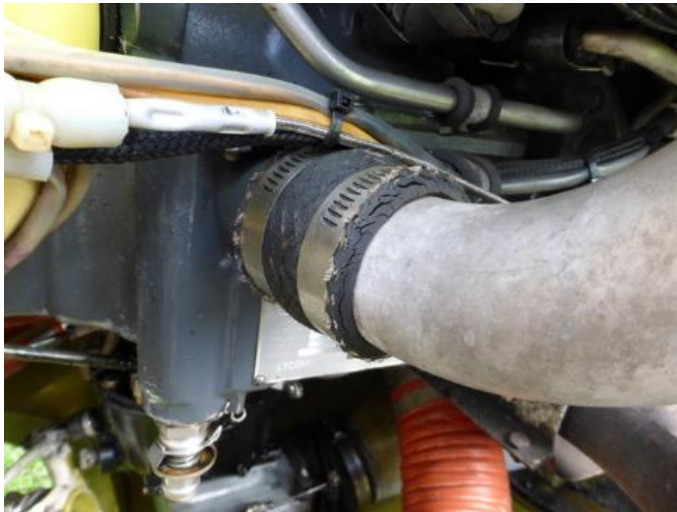
Illustration 3: Cracked rubber sleeves on the manifold pipes to the cylinders
